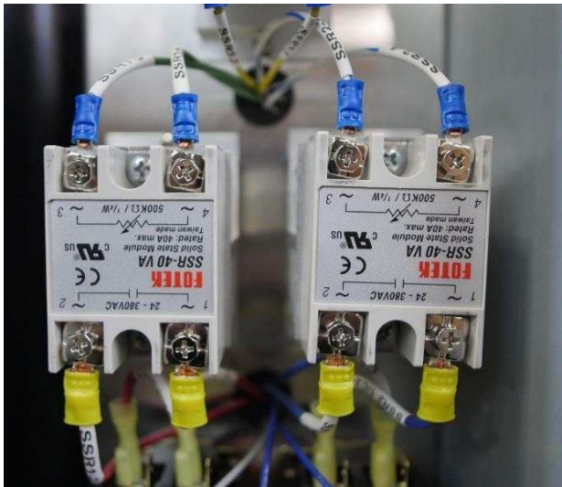
← SSR 1 and 2 Heat Control Modules
