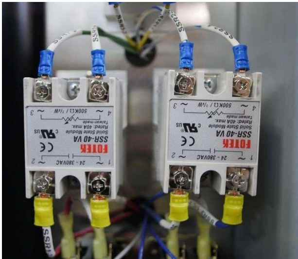
← SSR 1 and 2 Heat Control Modules
