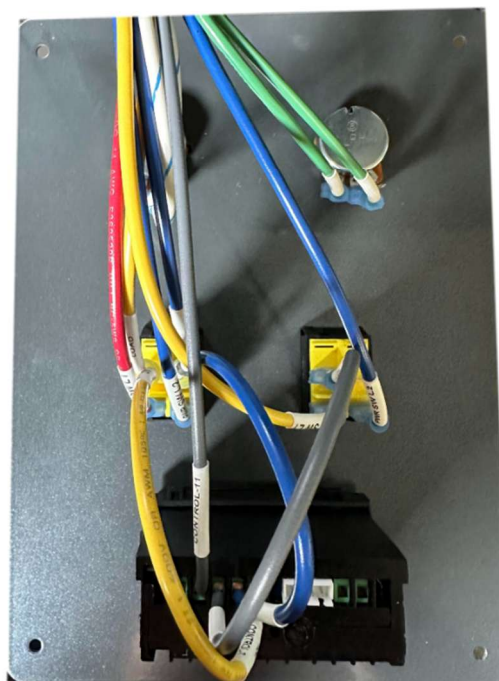
Figure 1.2 — Controller Wiring Beneath the Lid
