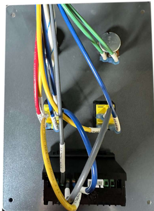
Figure 1.2 — Controller Wiring Beneath the Lid
