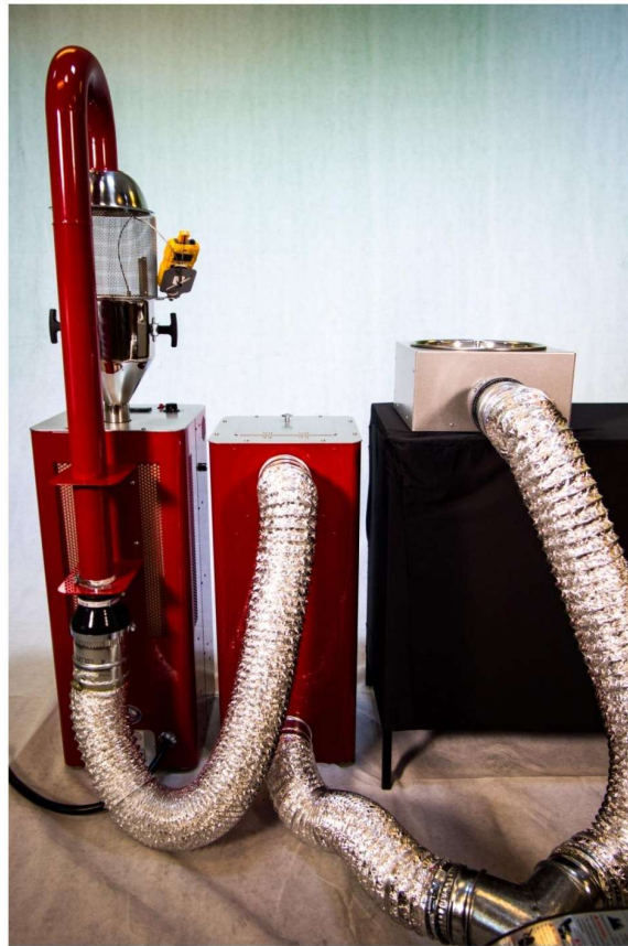
Indoor chaff collector installation
