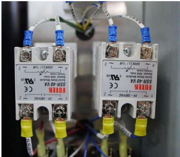
← SSR 1 and 2 Heat Control Modules
