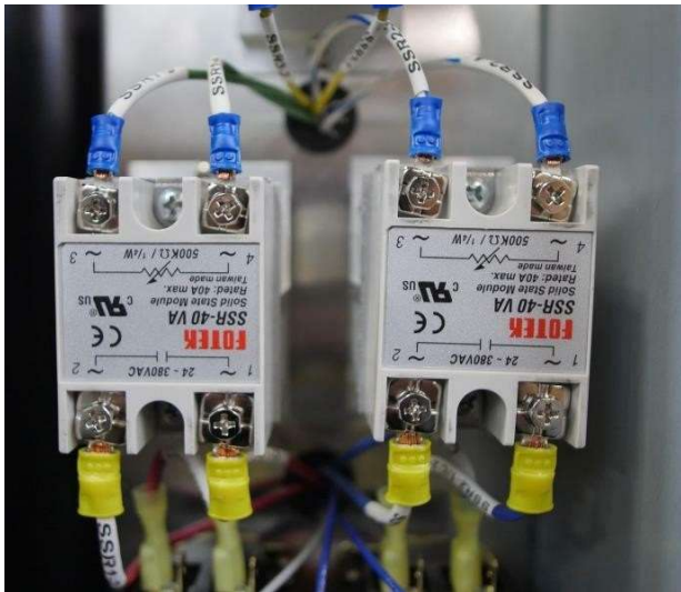
← SSR 1 and 2 Heat Control Modules
