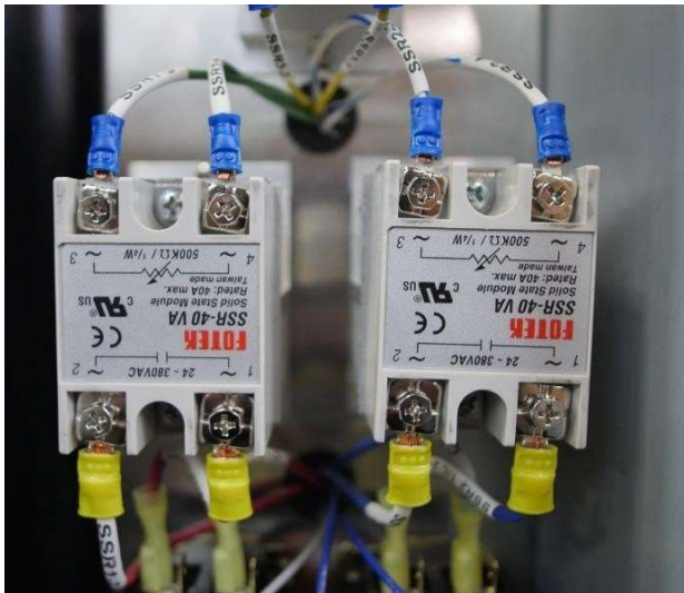
← SSR 1 and 2 Heat Control Modules
